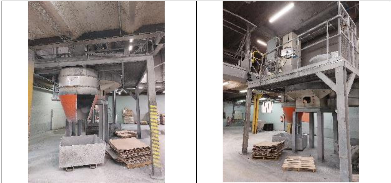
Figure 4: Mixing equipment - left: discharging area / right: mixing area
